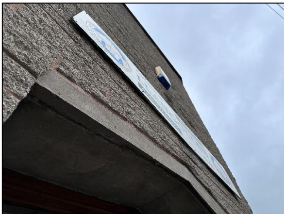
Figure 8: Voids behind the signage.
