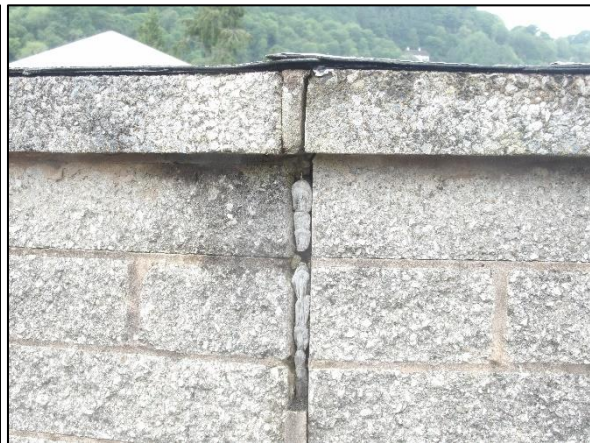
Figure 7: Minor voids in the stonework.
