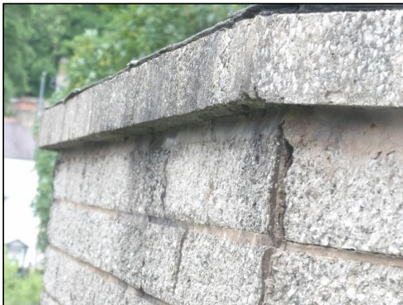
Figure 6: The pointing around the coping stones.
